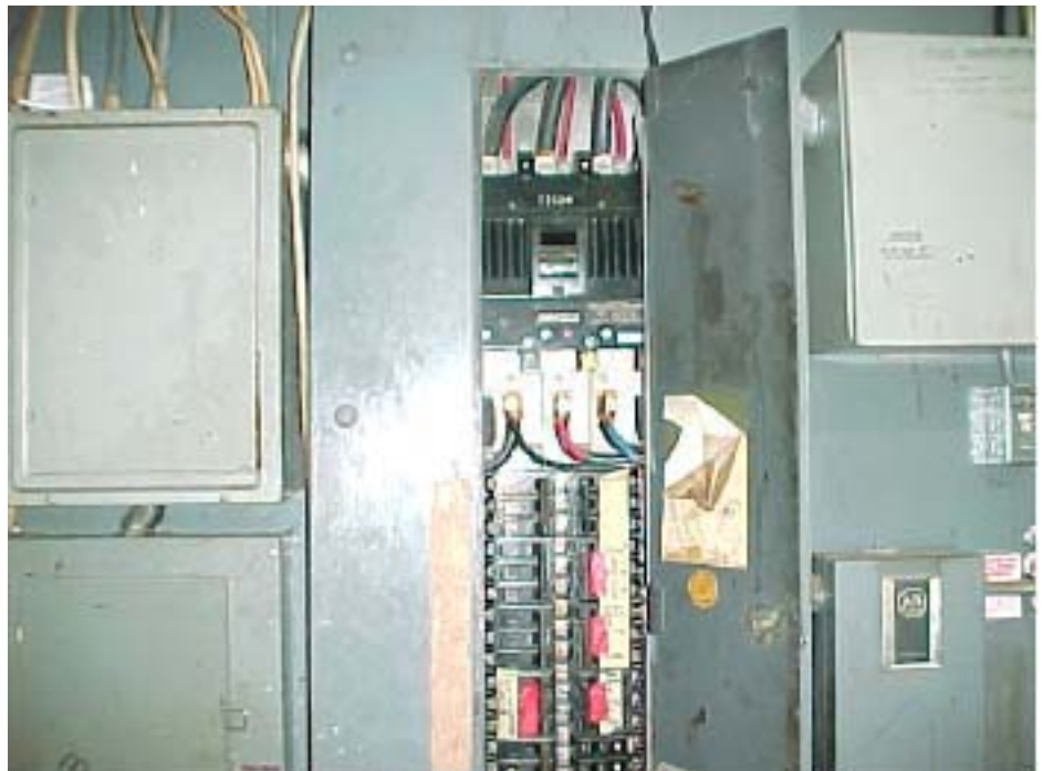
Typical Electrical Distribution Panel
