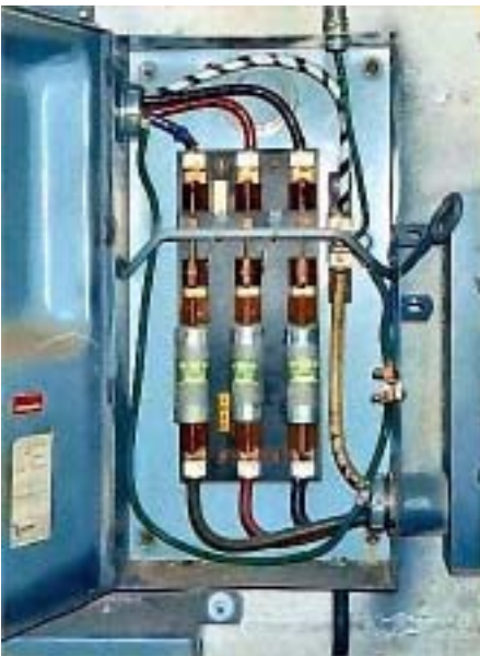
Typical Electrical Main Panel
