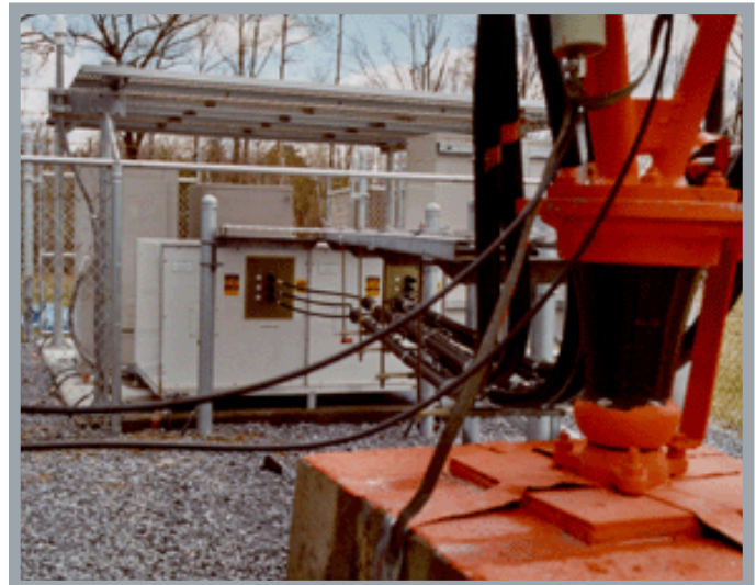
FIGURE 5: Cellular Collocation System On AM Tower
