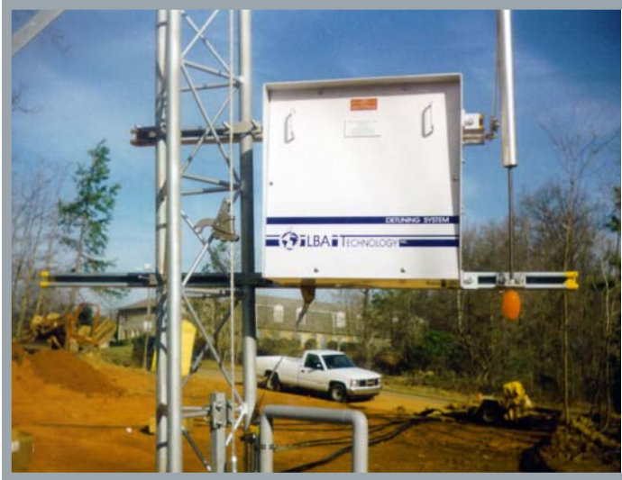
FIGURE 4: Cell Tower Detuning System
