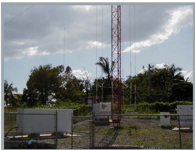
FIGURE 2: 10 Kw AM Triplexer Installation
